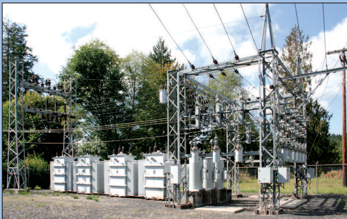
WOEC's Vernonia eastside substation is one of the co-op's substations that was built in a flood plain and will need to be replaced, a rate consideration for the future.
