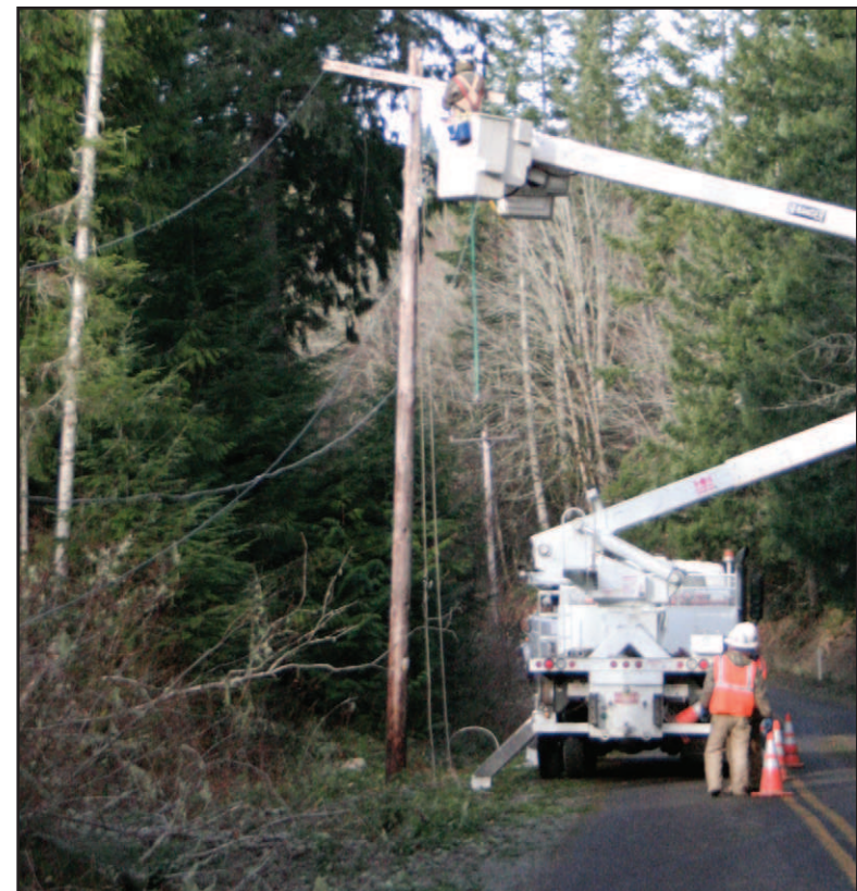
Another scene that was replayed all around the area after the recent storm is this one of linemen working on downed wires.
