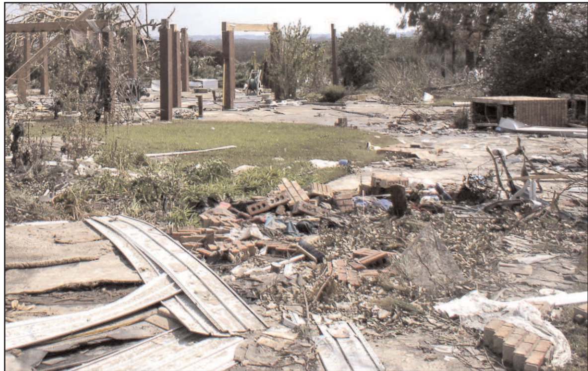
All that is left of the Biloxi home of Craig and Carolyn Wagner are pilings and rubble.
