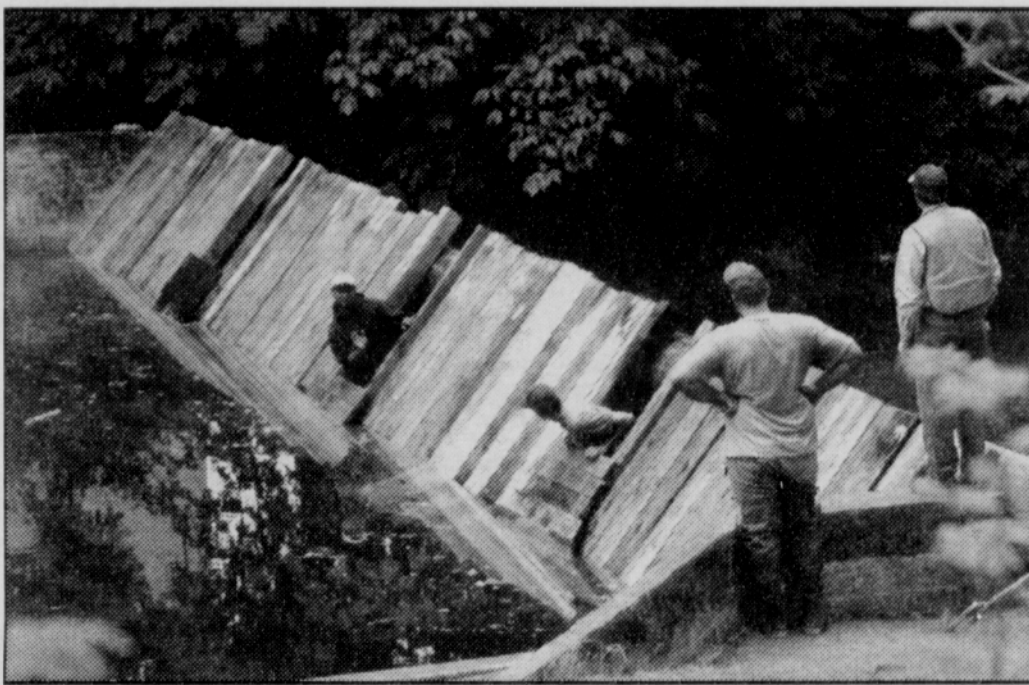
The annual raising of the dam, to create Dewey Pool for the summer, took place last week thanks to the Public Works employees shown above caught in the act.
