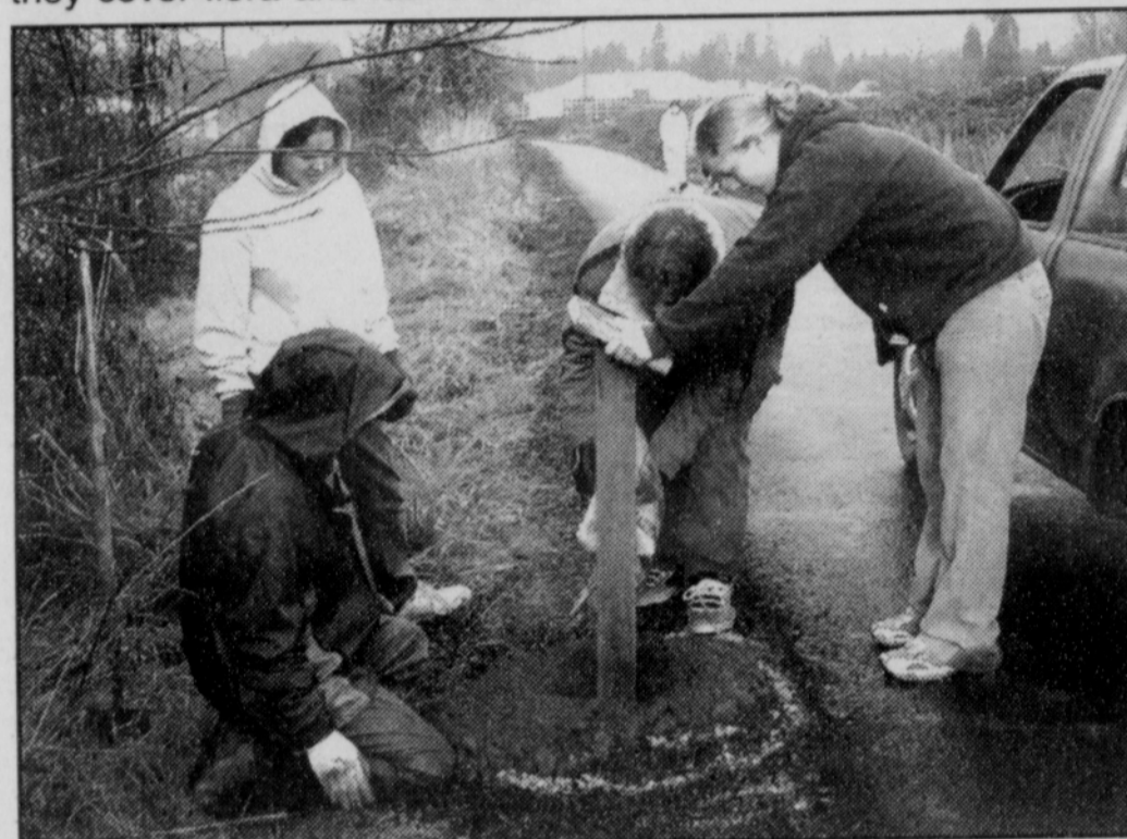
From left, Scout Master Patrick Peets, Elizabeth Brookins, Torin Tierney and Laura Brookins set posts as part of Tierney's Eagle Scout project, installing interpretive signs around Vernonia Lake and along Webb Way.
