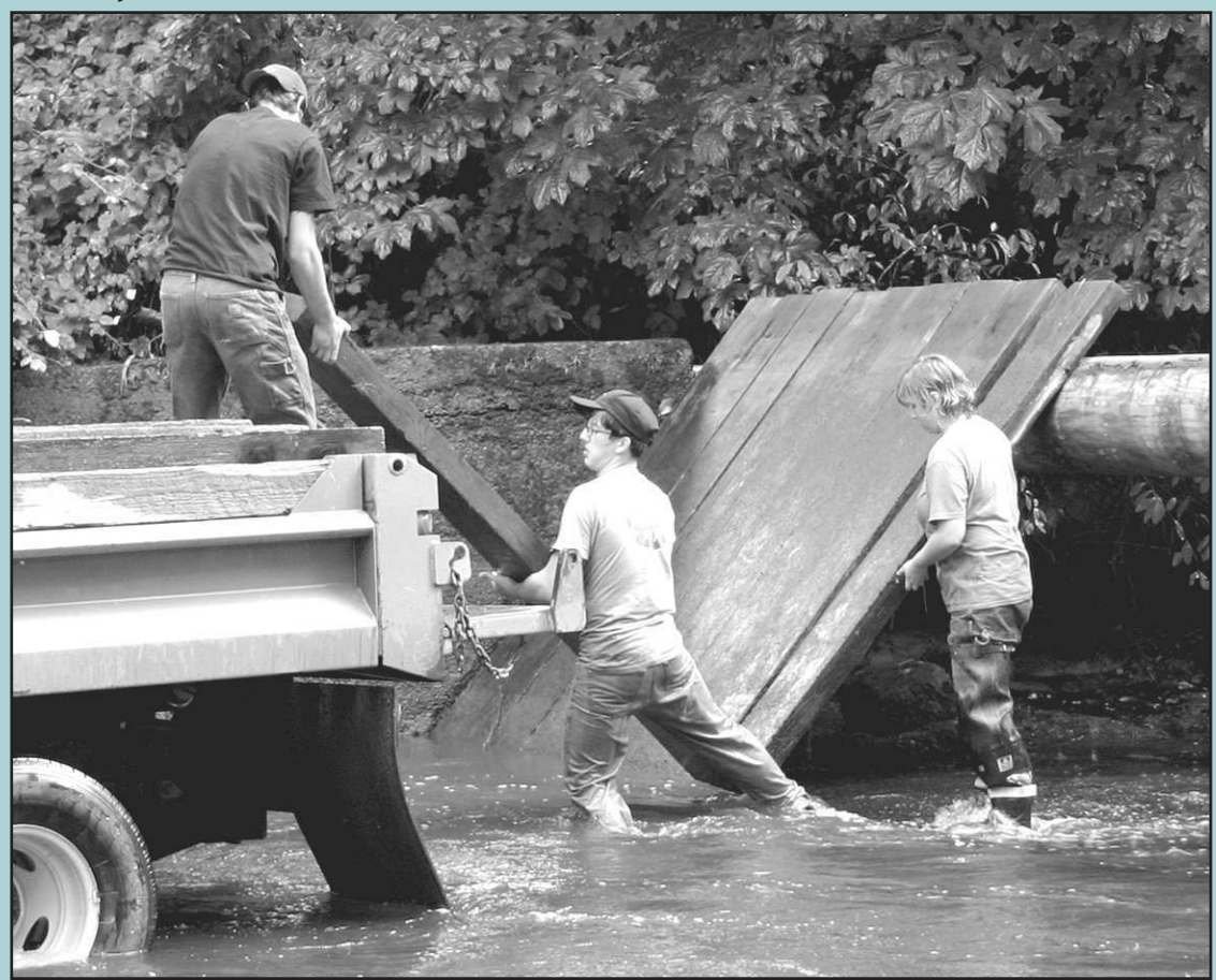
When heavy rains induced salmon to start upstream earlier than usual, OYCC members Brian Cook, Christopher Richardson and Keri Anne Johnson moved quickly to remove the planks that help dam Rock Creek for the swimming pool.
