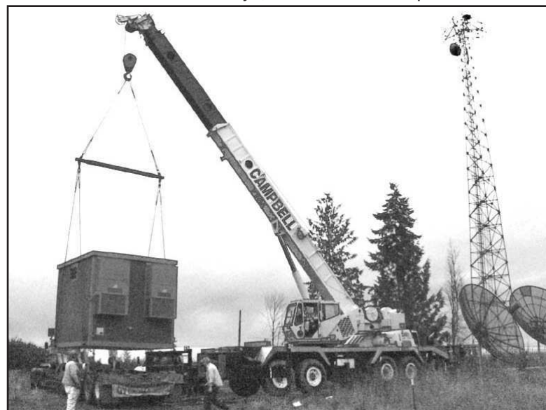
A building needed for the microwave communications system was delivered to Corey Hill in December, before ice and snow temporarily halted progress.
