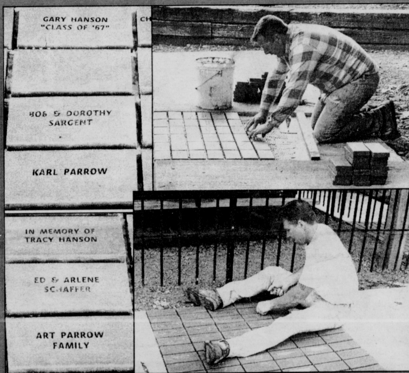
Loren Dennis, top, has been spending his spare time doing the same thing he does when he's working...setting bricks, with the assistance of Nathan Carrier, who is shown covering the engraved bricks with tape so the cement grout doesn't fill the engravings. At left are some of the engraved bricks. Engraved bricks can still be ordered; see article below for information.
