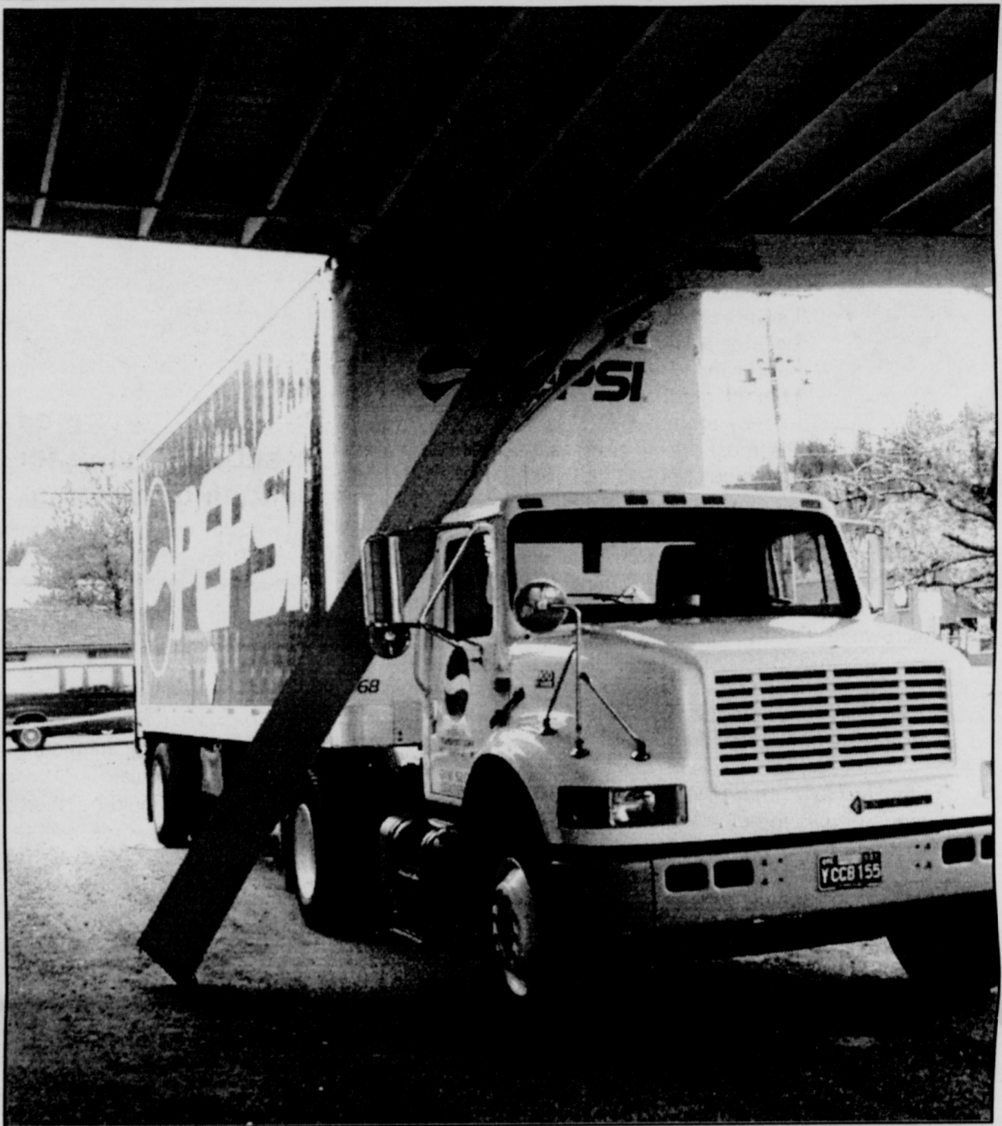
It was no contest when this Pepsi truck met a 50 year old canopy on the east side of Vernonia High School. The driver was new to the route and apparently was unaware that there was any other way to get to the parking lot.
