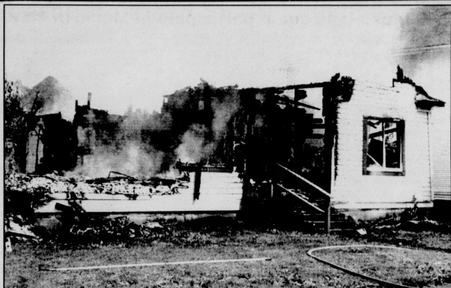
In December, when this North Street home burned, it was a tragedy that left a family homeless. In May, with the family's needs taken care of, the partially burned home became a training ground for Vernonia Rural Fire District volunteer firefighters as the home was alternately burned and extinguished.
