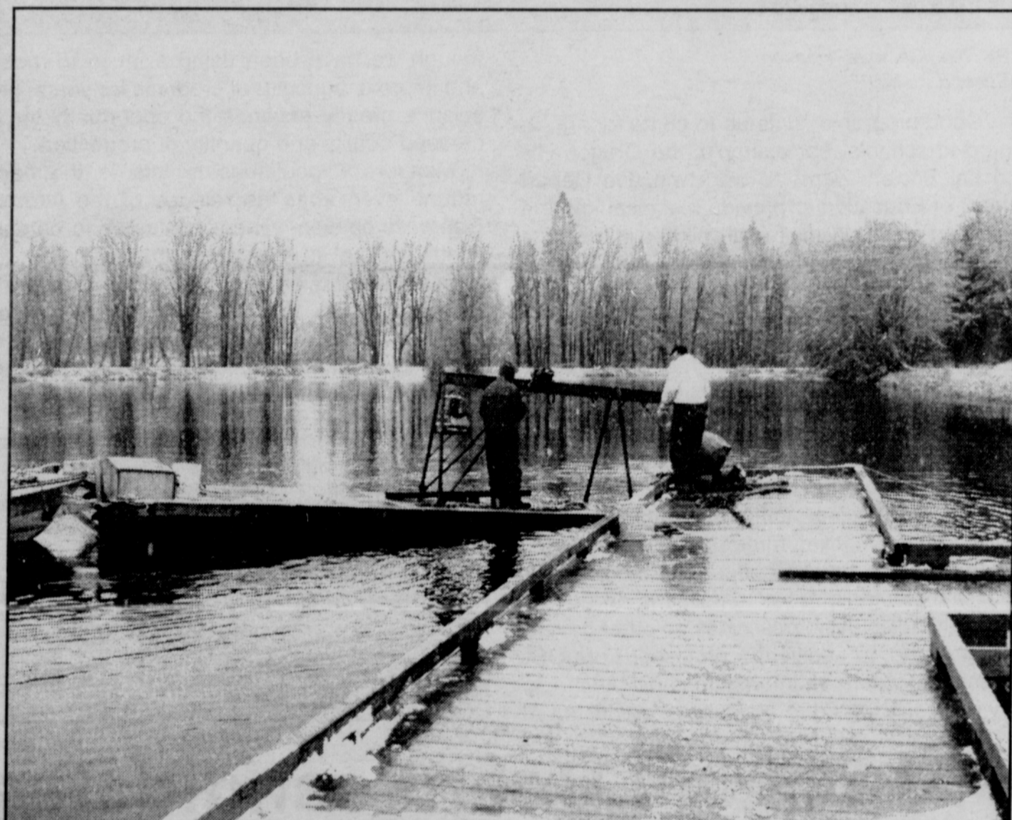
Cold wind and a little snow didn't prevent the installation of two floating piers on Vernonia Lake this month. The piers are handicapped accessible and will allow people with limited agility an opportunity to get safely out on the lake.
