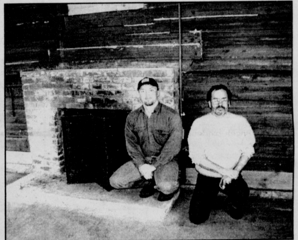
Moby Pendergrass, left, and Gary Pendergrass have been doing restoration work on the deteriorated logs in the Banks Log Cabin. Gary Pendergrass owns A Place in the Sun Log Homes in Timber.
