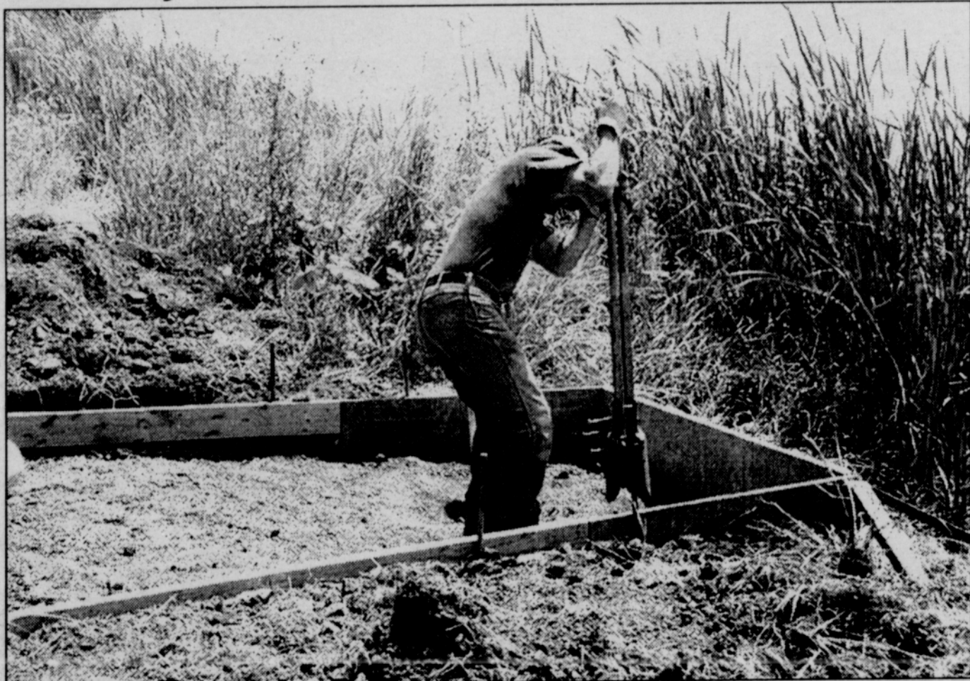
Dale Webb leans into preparations for a floating pier at Lake Vernonia. Concrete will be poured into two forms to use as "anchors" to attach handicapped-accessible fishing piers. One pier will be built on the east side and one on the west side of the lake.
