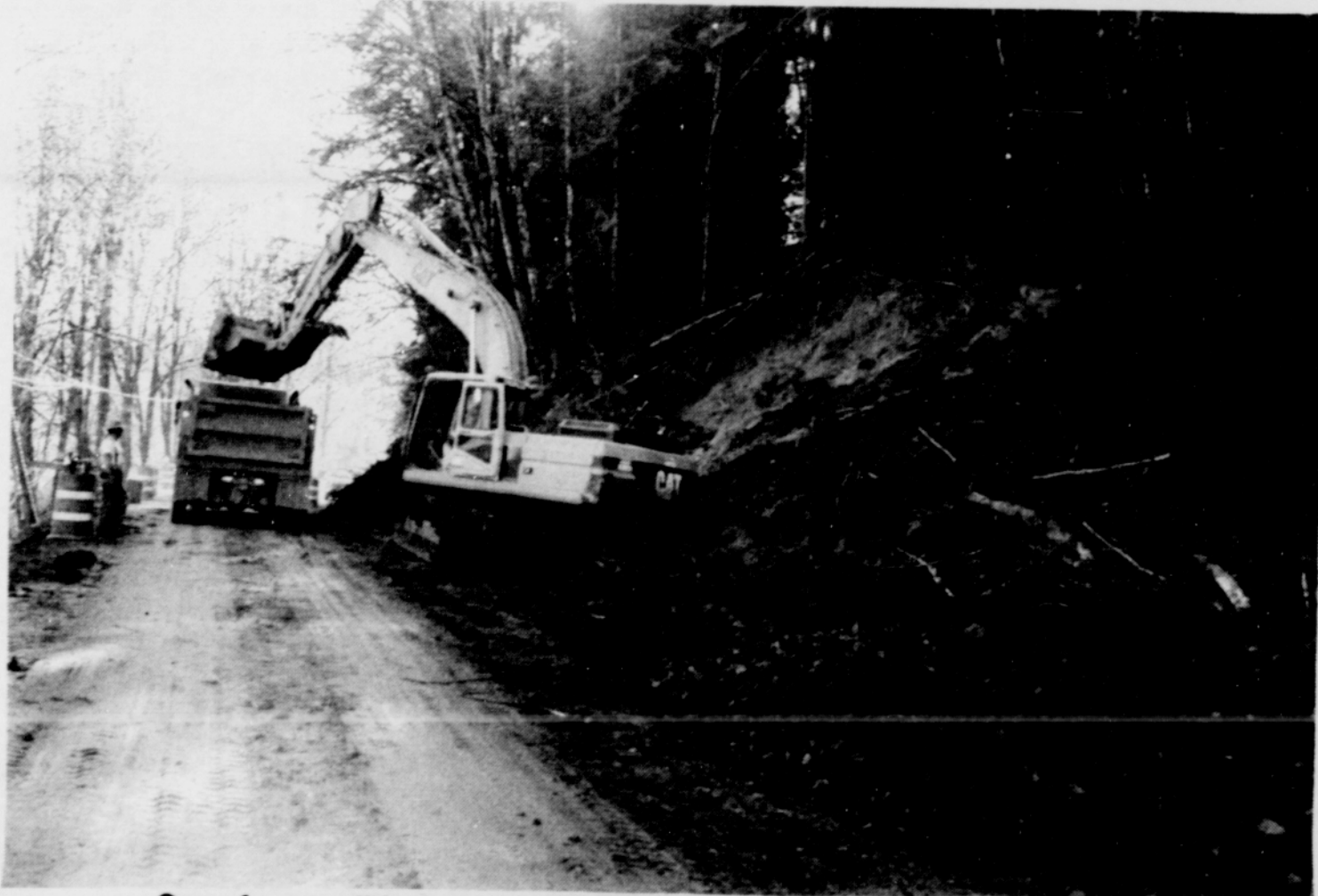
One of many slides on Hwy. 47, this one was north of Vernonia.
