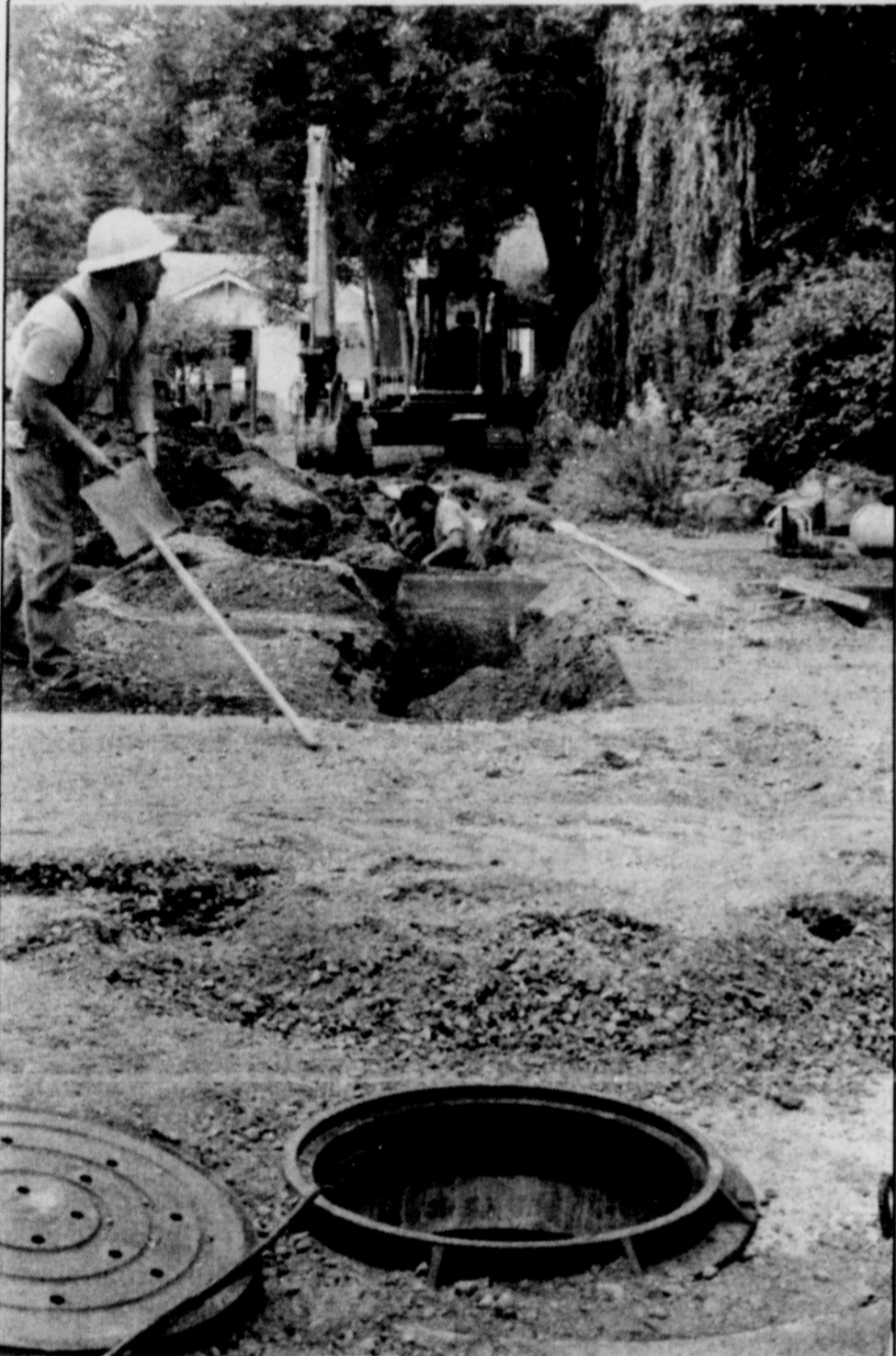
Dallas contractor J. W. Fowler is installing storm drain system on A Street.
