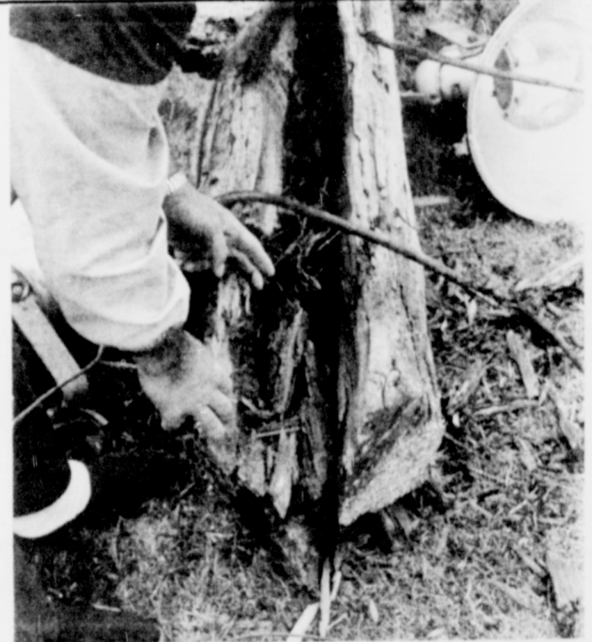
Extensive dry-rot is seen in one of the cross bars holding the VHS football field's lights, as well as in the top portion of the pole.
