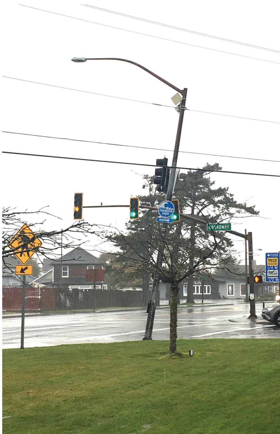
High winds disabled the traffic signal at the intersection of Roosevelt Drive and Broadway on Monday.
