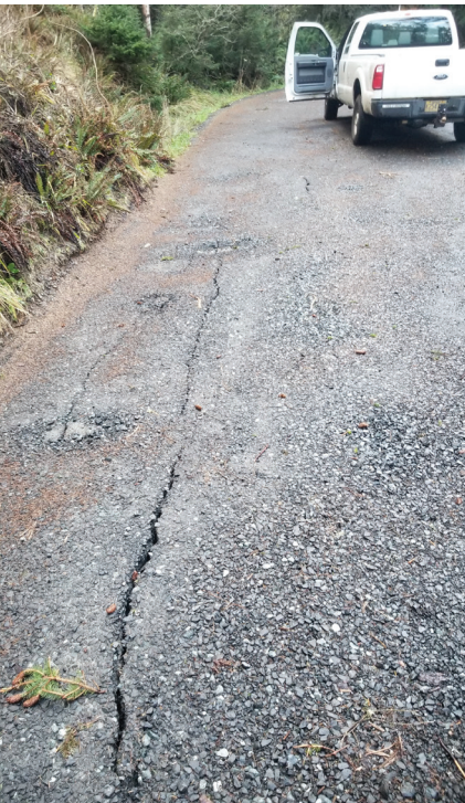
Road fissure at Ecola State Park.
