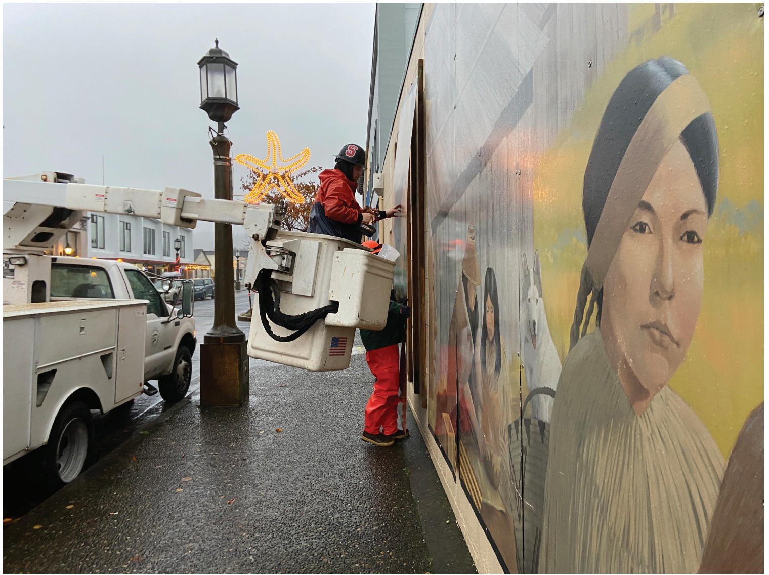
Seaside Public Works team removes sections of the mural on Broadway for repair.
