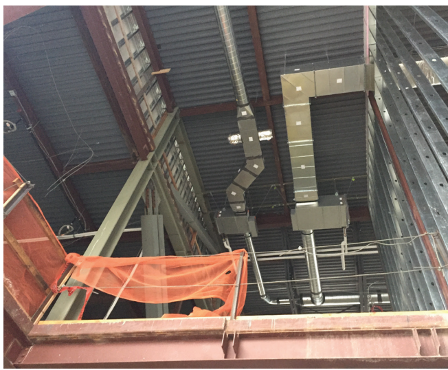
Duct work in the middle and high school building.
