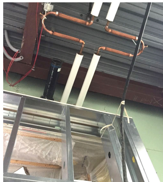
Pipes connecting the middle and high school are designed and clad to withstand seismic events.
