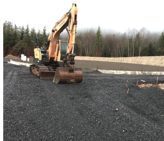
Above the high school and middle school, the city is building a reservoir to serve the school and surrounding residential area. This will be the highest elevation of the city's three reservoirs. In coming weeks the city contractor will be pouring a tank foundation and completing the north transmission line to Sunset Hills.
