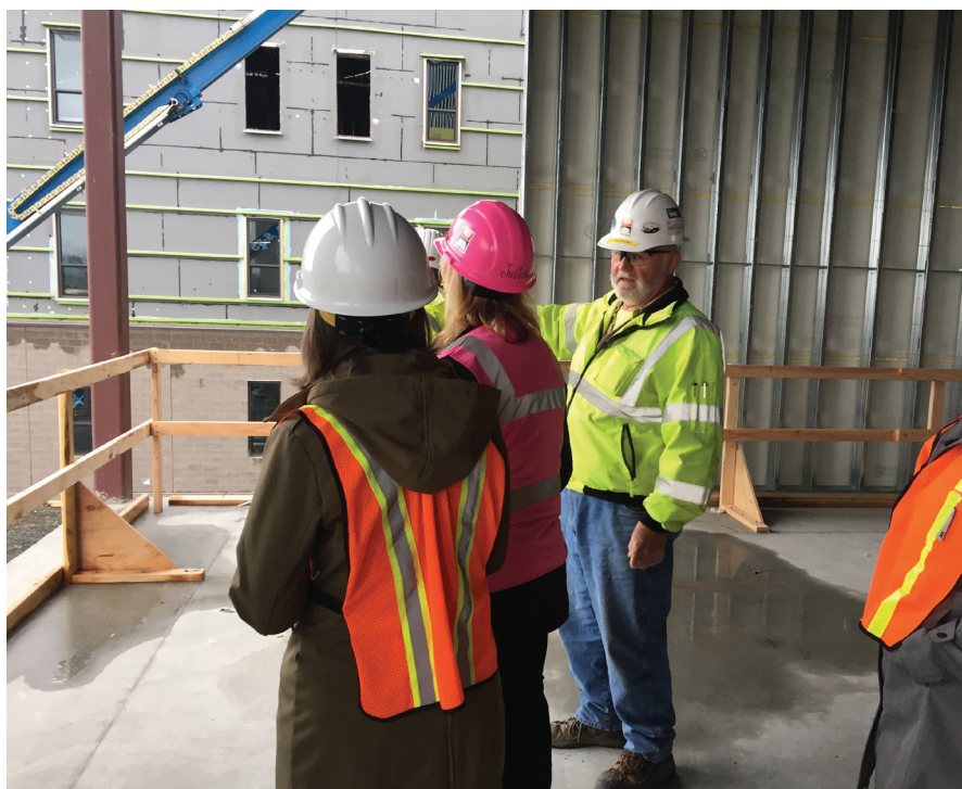
Phil Broome of Hoffman Construction leads a tour of the new site.
