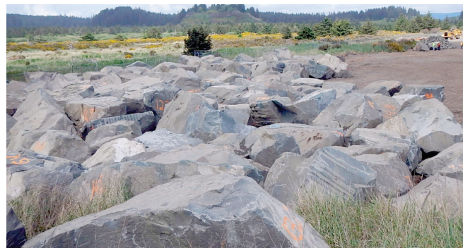
USACE/Ed Saldan The U.S. Army Corps of Engineers is staging equipment and material to repair the 100-year-old navigation structure.
