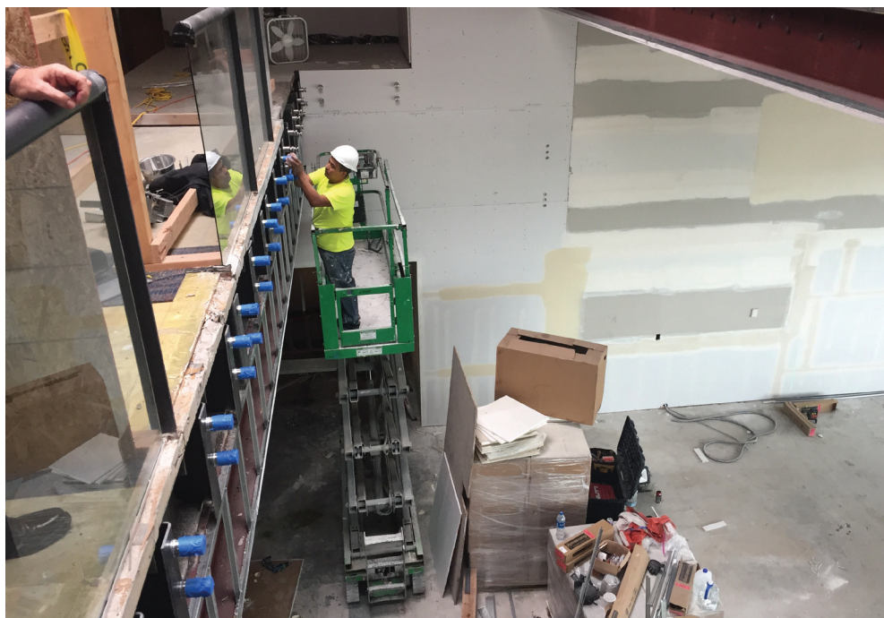
Construction worker in the main lobby. Work is expected to be completed at the end of the month.
