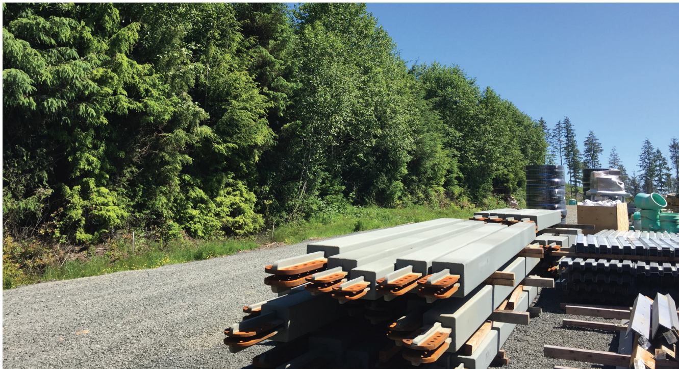
City crews will soon begin work on a reservoir tank in the East Hills.
