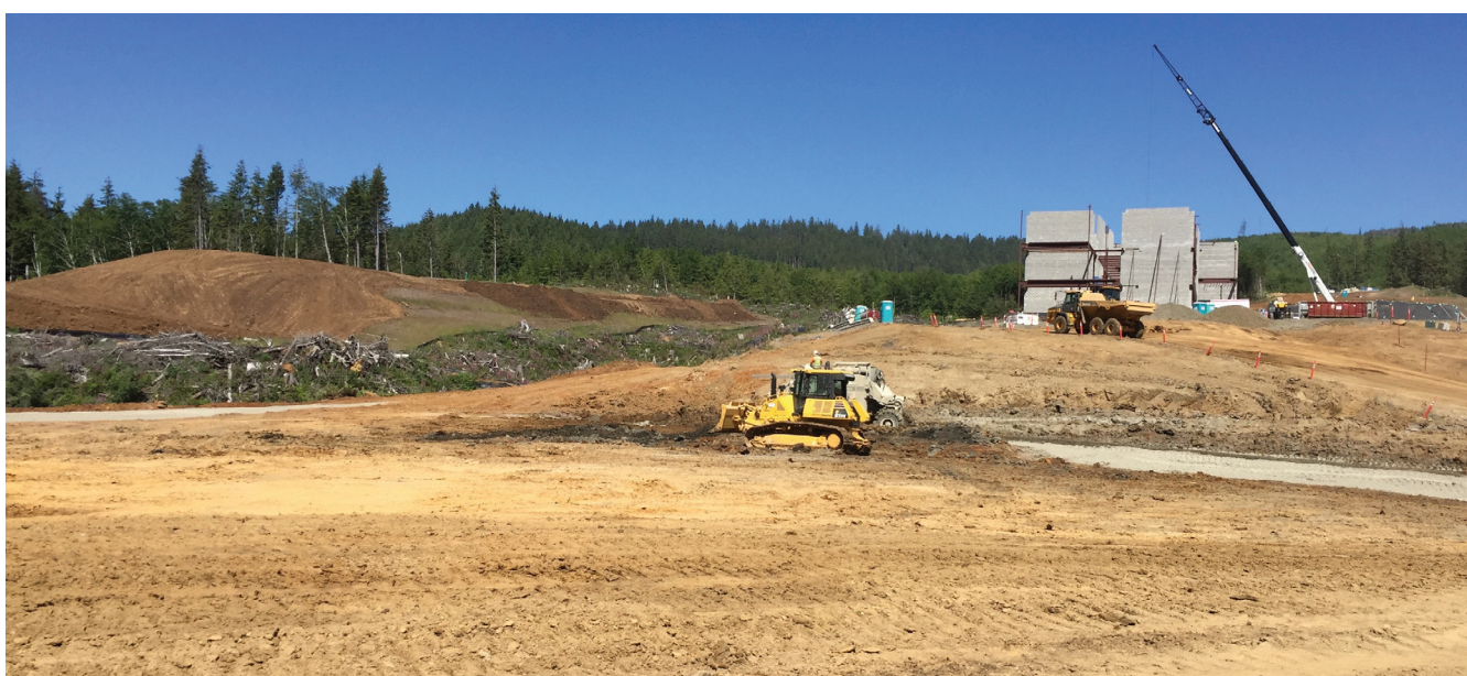
Work on athletic field at the new middle and high school campus.
