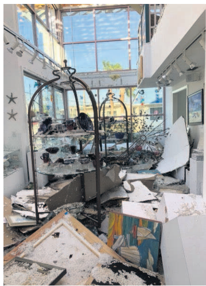
Damage at the Paul Brent Gallery after the hurricane that hit in Panama City, Florida.
