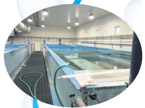
Inside the city's water filtration plant.
