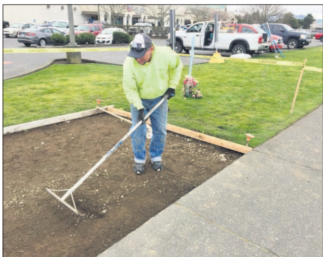
Contractor Eric Huntsman at work raking the area of the bus shelter in Seaside.
