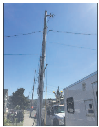
Cable must be removed from wires before poles can be taken down.
