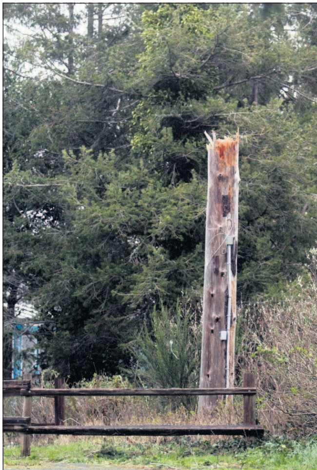
This pole snapped in a storm, causing the destruction of the osprey nest.
