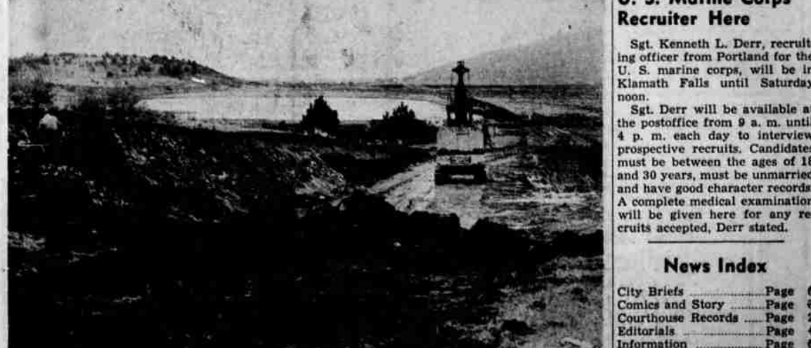
Work recently started on the newest cutoff under the state highway department's road straightening plan for The Dalles-California highway was being pushed forward this week despite unfavorable weather conditions. The new route, which will eliminate the present stretch through Wocus, will be approximately four miles in length.
