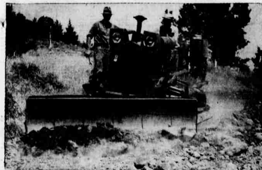
This bulldozer, manned by a state forestry department crew, is shown at work on the Old Fort Klamath road east of town, from where a firebreak is to be built along the crest of Hogback to Olone. The first job done by the crew has been to put the Old Fort road into shape so that a fire fighters' truck, carrying a tractor, can get over it into brush and grass country beyond. A short piece of the Swan lake road will also be worked over, and the construction will begin on the firebreak, proper. The county has improved the Old Fort road from the city limits to the place where the forestry crew took up the job.
