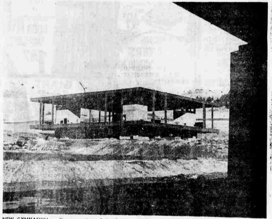
NEW GYMNASIUM — The gymnasium of the Oregon Technical Institute campus is shown in this photo. Each of the four pillars in the building contains a staircase to the upstairs gymnasium. The gym and the rest of the new campus northeast of Klamath Falls is scheduled to be finished by next fall.
