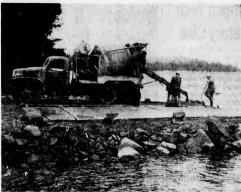
NEW RAMPS AT DIAMOND LAKE — Forest Service crews finish pouring concrete for new boat ramps at Diamond Lake, visited by nearly 110,000 vacationists this summer. Funds for the program were obtained through the Accelerated Public Works Program.
