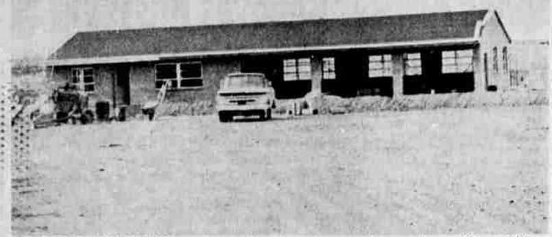
REFUGE CONSTRUCTION — A machine shop, storage shop, and an office building and garage, pictured, are three new buildings under construction on the Modoc Fish and Wildlife Refuge. The project will cost an estimated $80,000.
