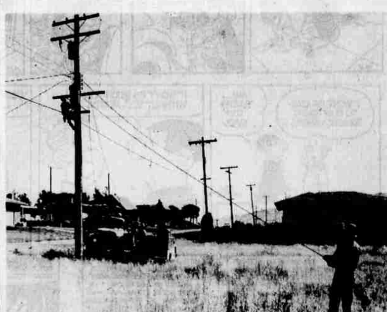
WORK MOVES AHEAD — A new transformer is raised into place in northwest Klamath Falls where Pacific Power and Light Company local crews are increasing the capacity of distribution circuits from 4,100 to 12,500 volts. This is part of a program to provide added capacity to the city's distribution system to meet increasing power demands here. Work on the entire voltage conversion program will be completed by the end of the year.
