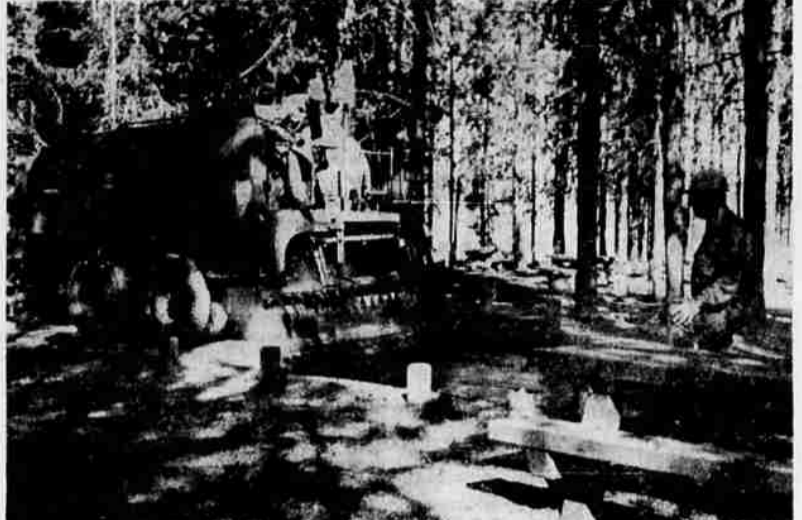
PAVED ROADS TO SERVE CAMPGROUNDS — Tom Hollaman, district road inspector, observe workmen apply the first coat of oil on a camping spur in the Diamond Lake Campground. All roads into the national forest facility are being paved this fall. —U. S. National Forest Service photo
