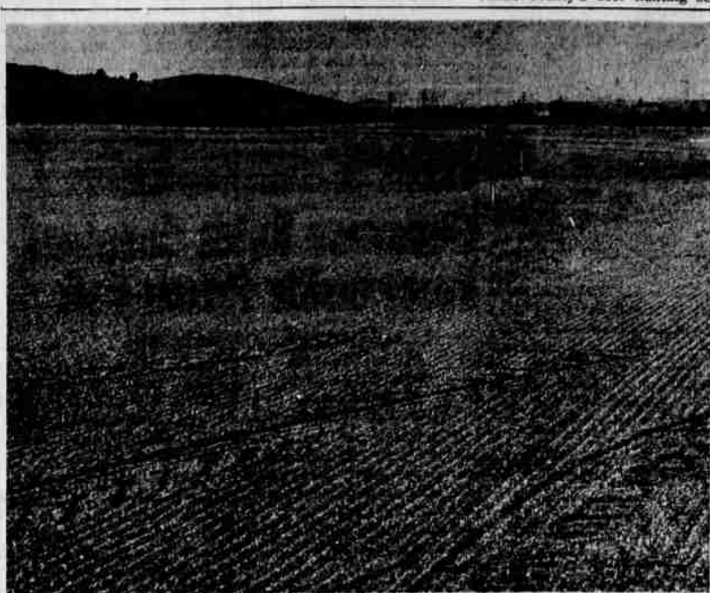
PARK SEEDING —Grass seeding on this portion of Kit Carson Park in Klamath Falls is being completed by city crews of the Department of Parks and Recreation. This area, shown covered with sawdust to protect the seed, will eventually become a baseball field. An automatic underground sprinkler system is also being installed with the seeding.
