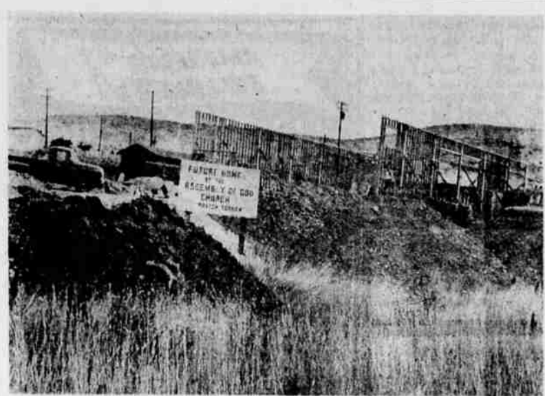
CONSTRUCTION PROGRESS — Under construction for seven weeks, the future $75,000 home of the Assembly of God Church is beginning to take shape on Alameda Avenue. The new church has been in the planning stages for approximately three years, with the property purchased in 1960 and the ground-breaking service held last March. Expected to be completed by the middle of next summer, the frame and rock structure will have a capacity of 500. Rev. Lloyd F. Fosner is the pastor.
