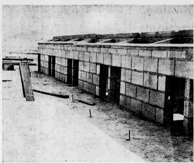
NEW KENNELS BUILT — Photo shows new kennels being constructed at the Klamath Falls dog pound on Memorial Drive. Ten new kennels will double the capacity of the pound. The kennels feature built-in heating and are constructed of concrete. The construction will allow five temporary kennels to be demolished.
