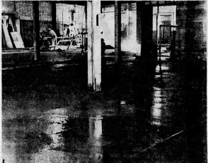
FLOOR POURED FOR POST OFFICE — Photo shows the still-wet three-inch concrete floor poured in a Klamath Avenue garage, which is being converted into a temporary Klamath Falls Post Office. The interior of the garage is being remodeled for Park and Shop Corporation, which is leasing it to the post office. Postal employees will move into the garage the middle of next month and will be housed there for about a year while the main post office building is expanded.
