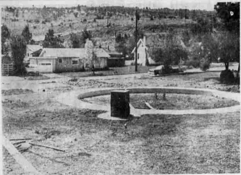
PLAGROUND SANDPIT — This ring of concrete will enclose a sandpit at the new Richmond playground, which is under construction by the Klamath Falls Department of Parks and Recreation. In front of the pit is a water fountain. The playground at Second and McKinley streets is costing about $4,000 to develop.
