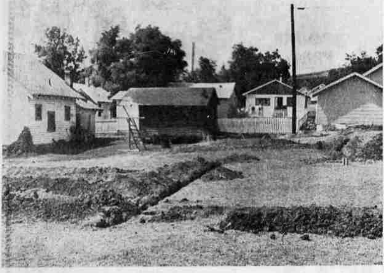
IRRIGATION SYSTEM — These trenches at the new Richmond playground, Second and McKinley streets, will enclose the first automatic irrigation system to be built into a city park. The half-acre playground was once a weed-choked lot, but city crews have been working on the site for the past several weeks.
