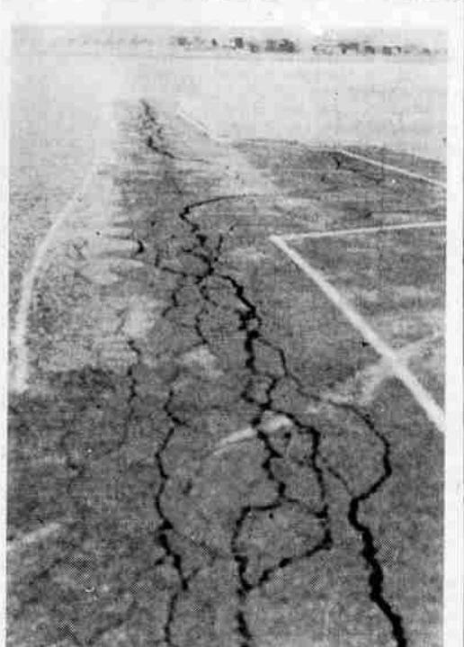
CRACKS ON AIRPORT RUNWAY — These are some of the 43,000 feet of surface cracks that will be repaired by the City Street Department at the Municipal Airport starting this week. The State Board of Aeronautics has agreed to defray 50 per cent of the $24,000 estimated cost of the project. Some of the major repairs will include complete removal and replacement of some of the worst sections and reinforcing the sub-base. Work on the runways is expected to last over a month.
