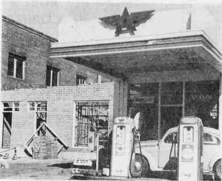
FILL 'ER UP — Work is progressing on the Tidewater Associated Flying A Service Station at Fourth and Main owned by E. D. Peterson. Peterson has been in business at the same location for six years. The new station replaces an outmoded structure. Cole Construction Company, Portland, is the contractor. Majority of subcontractors are local. Benjamin F. Lambert and Sons have reopened a Flying A station in the motel district of Wocus that has been closed for a year.
