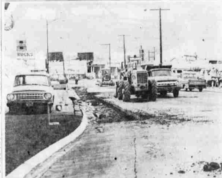
STREET BEING REPAIRED — This section of Klamath Avenue, stretching from Eleventh to Commercial Street, has been blocked off to enable the street department to tear up portions, replace the base and eventually resurface. Paul Hamblin, street department superintendent, estimates the street will be closed for another week. This view was taken from the corner of Eleventh and Klamath.
