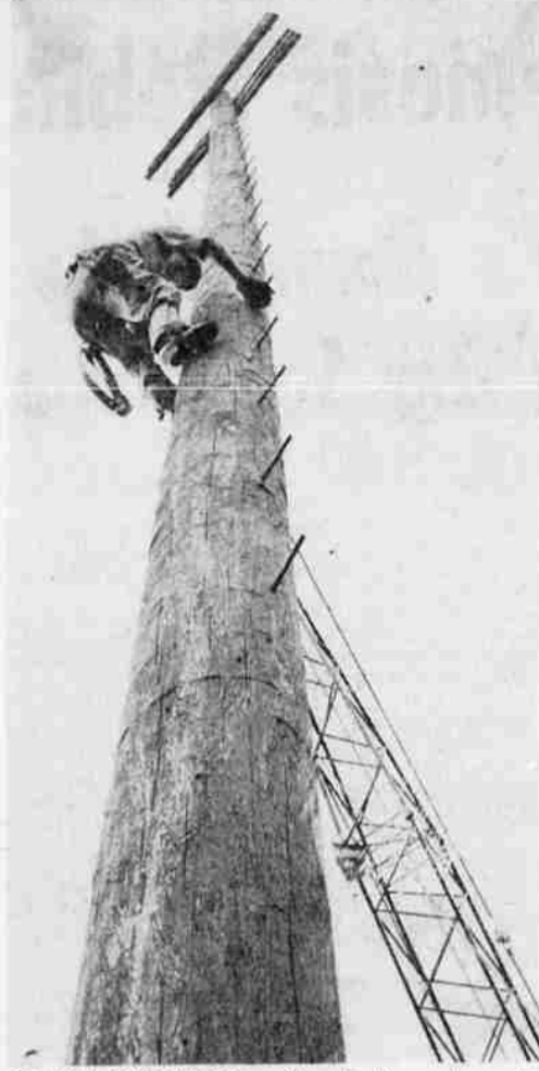
GETTING FACE LIFTING — Gem Stadium got a partial face lifting this week when two new sets of 90-foot poles were put up at the stadium to aid the lighting system there. These 90-foot poles, four of them in all, were placed upright by a huge crane. A worker climbs the pole to prepare it for lines and the lights.
