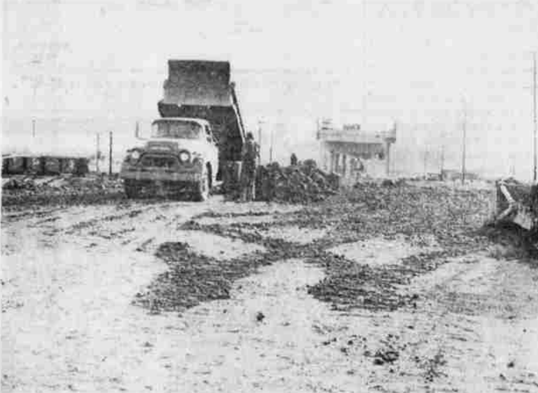
GRADE BUILDING BEGINS — A great deal of grade building will be necessary before this elevated overpass can be used by traffic. The concrete overpass spans the Great Northern tracks on Washburn Way. The road bed is being constructed by the Klamath County Road Department. It is estimated that it will take 109,000 cubic yards of fill to complete the project at a cost of about $150,000. About 18,200 truck loads of dirt will be needed to do the job.
