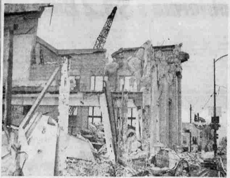
INDESTRUCTIBLE BUILDING — Progress is slow for the wrecking crew that has been trying for more than one month to batter down the walls of the old U.S. Bank building in Grants Pass. The 15 inch concrete reinforced by steel bars even knocked the "eye" off one 2,000 pound steel ball last week. —UPI Telephoto
