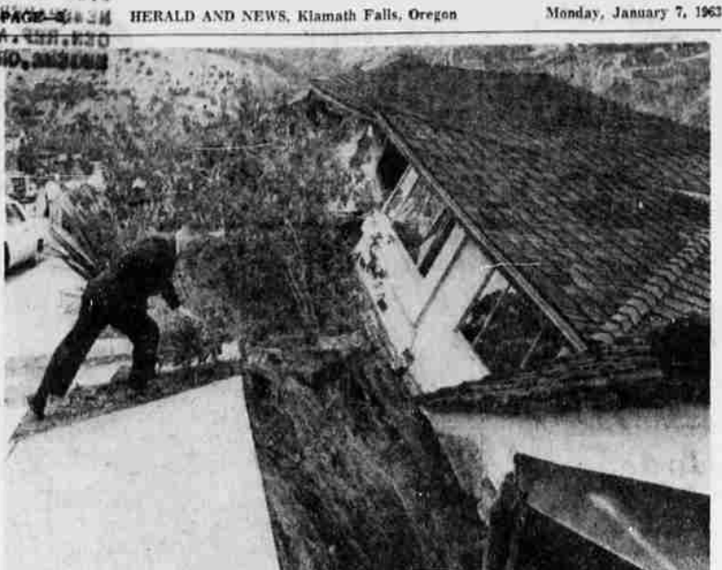
HOMES DEMOLISHED BY SLIDE — A Brentwood, Calif., water inspector uses caution as he peers from cliff-hanging sidewalk into gaping hole left when two homes were demolished due to landslides.
