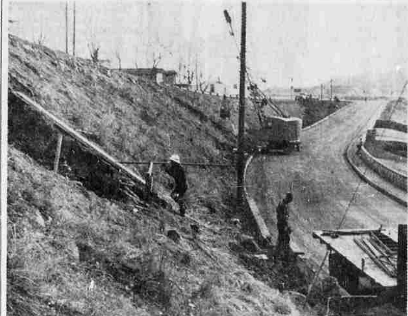
SOUTH INTERCHANGE WORK UNDERWAY — Construction work on the bridge that will span Lake Ewauna for the south interchange of the west side bypass is moving rapidly ahead. Besides the demolishing of a service station to make room for an off-ramp for southbound traffic, workers are busy getting ready to pour concrete pillars to support the bridge structure which will take off from about the top of the incline near Main Street. In this view, workers are preparing areas for pouring the supporting pillars. Tom Lillebo, Reedsport, has the contract. The State Highway Department listed the estimated cost of the project as $861,000, and completion date as April 1, 1964.
